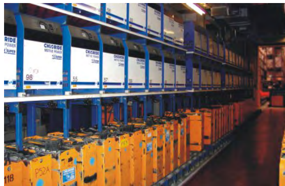
A Typical Battery Room
